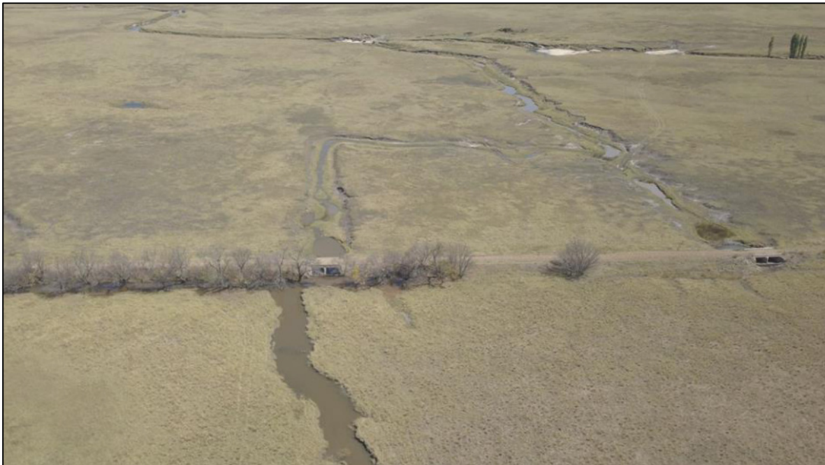
Plate 11-7: Aerial view of the railway and culvert crossings in the Flood Plain as well as the canalised water flow
