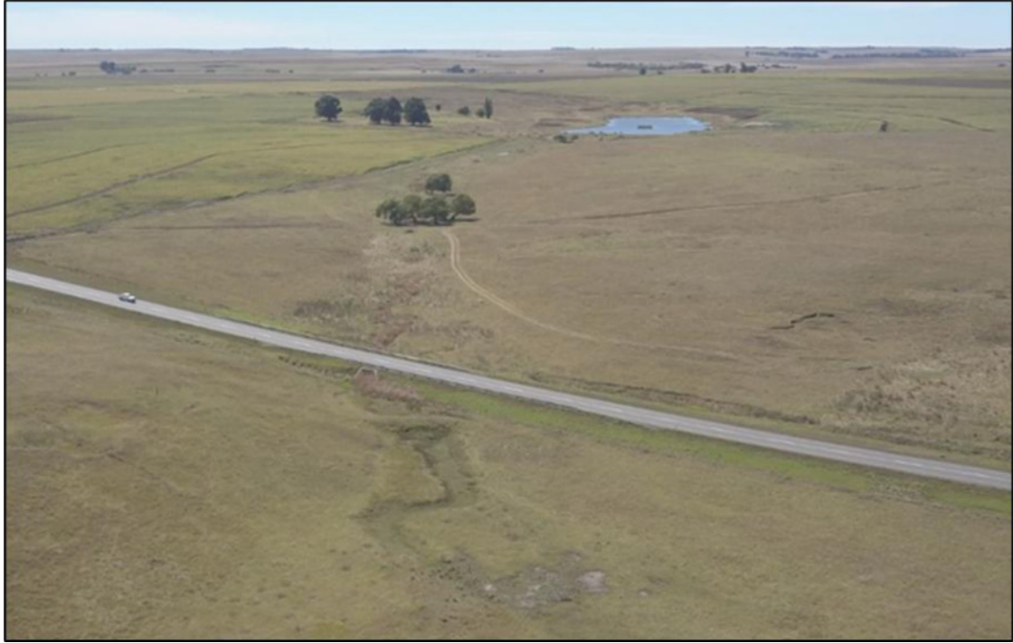
Figure 5-4: Aerial view of the culvert and road crossing the Seep as well as the dam and impoundment area
