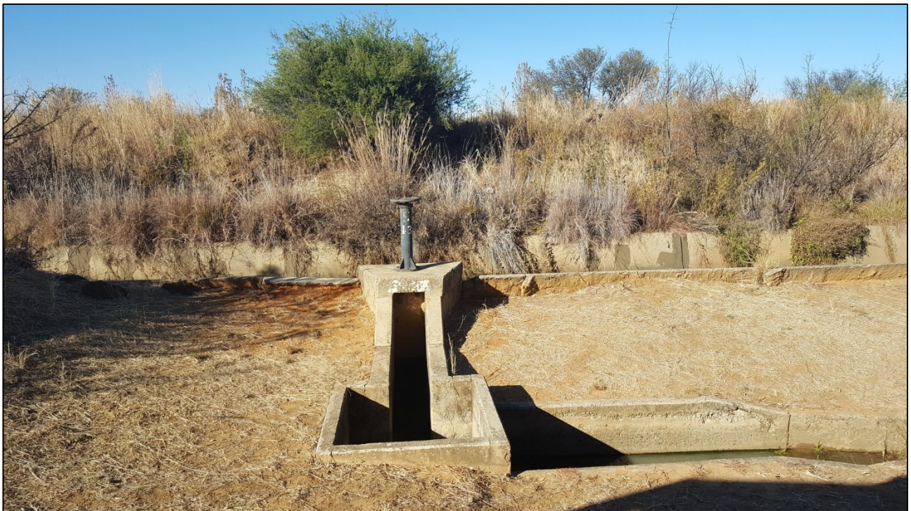
Figure 52 – Sluice-gate at canal, Site 014.
