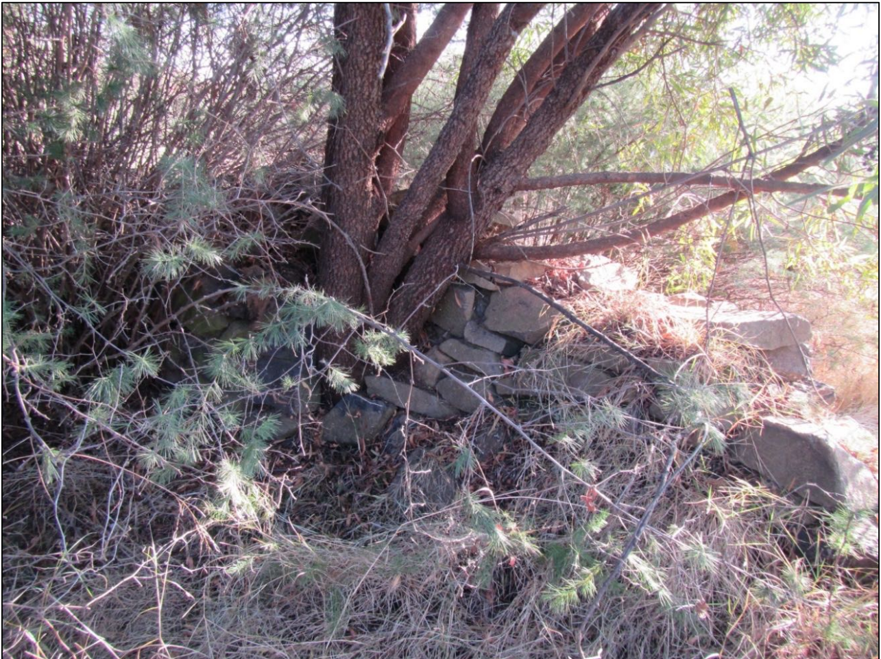
Figure 80 – Another view showing a tree growing through the wall.
